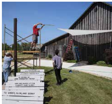
Shade sails were installed and Birch Creek's familiar benches received a fresh coat of paint in time for Opening Night on June 17. On stormy nights, summer interns lowered the sails and concerts moved inside the Dutton Concert Barn.
